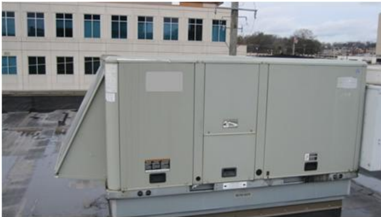
FIGURE 1 COMMON PACKAGED ROOFTOP UNIT
